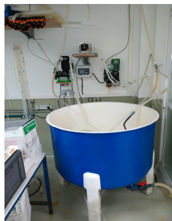
Figure 32 Cylindrical tank of 560 L for microalgae storage. Three pumps for feed distribution are set above the tank; an 8 channel peristaltic pump is set in the middle
