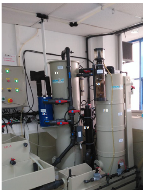
Figure 31 Seawater recirculation system (RAS) with reserve pond (BR), head tank (TC), biological filter (FB), heat exchanger (IC), "skimmer" (SK) and ultra-violet unit (UV)
